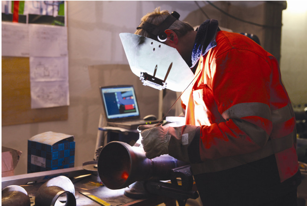
Figure 6 Welding of pipes directly from a virtual 3D model viewer. Image courtesy of Ramboll Denmark and Brøndum.
